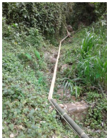
Giant bamboo protective shield for PVC water supply pipes
